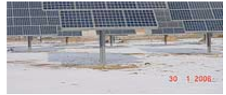
The 150 kW Villa de don Fadrique PV array, with trackers, in Toledo province GEA
