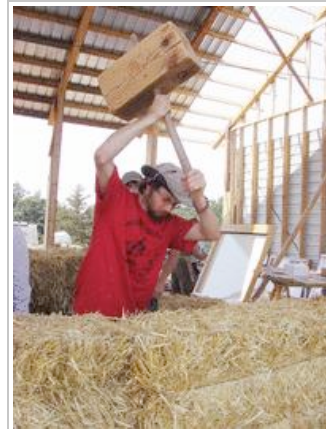
Lonnie Gamble Big Green Summer student Avi Pogel uses a custom wooden mallet to adjust straw bales during construction of Big Green Summer's new shop/lab, office and classroom building.
